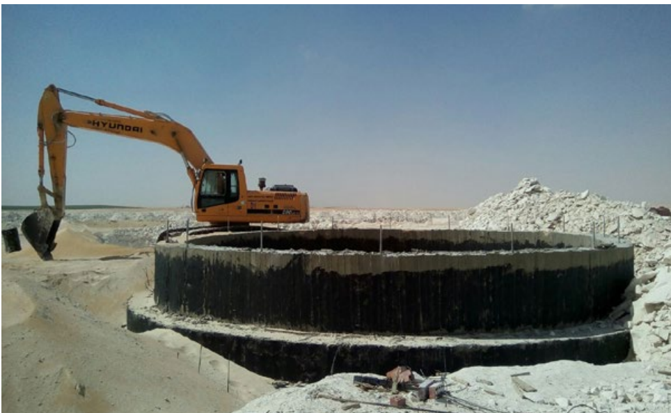
Farafra Diesel Power Station Farafra, Egypt
